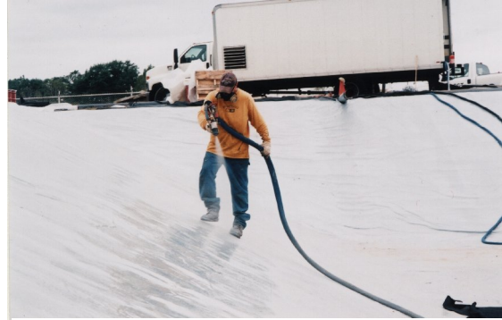
A typical construction/industrial-based application for polyurea includes ElastoGard ARC is sprayed onto geo-textile fabric as a wastewater pond liner. (Picture courtesy of Mike Francis-Protective Coatings)
