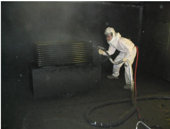
A typical O.E.M Polyurea application with proper spray booth and personal protective equipment.
