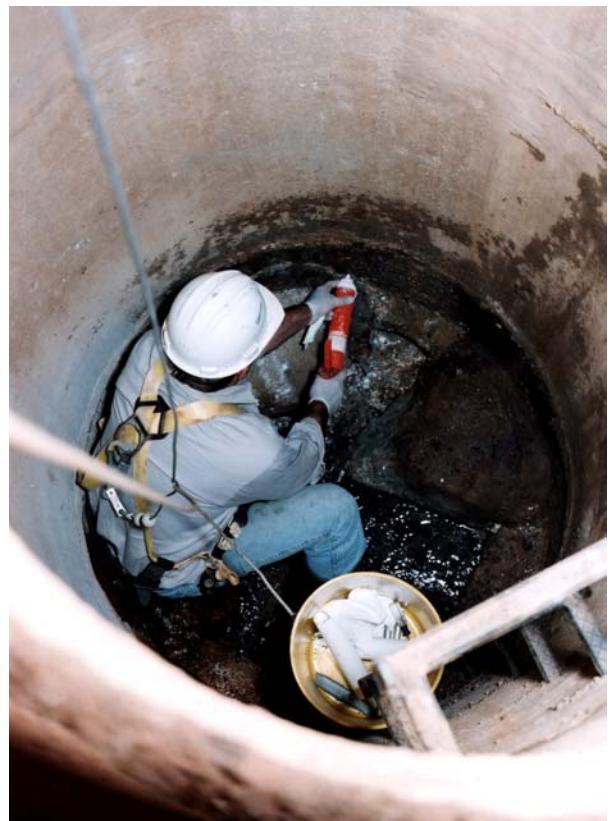
Mike Kronz of Remote Orbital Installations Preparing a Manhole for a Polyurea Lining
