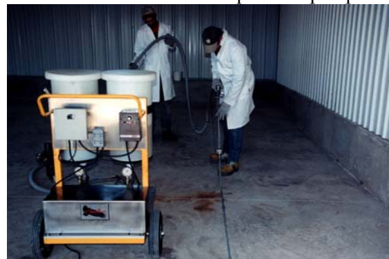
The ESI “Condor” Low-Pressure Dispensing Machine Being Used to Apply Polyurea Caulk
