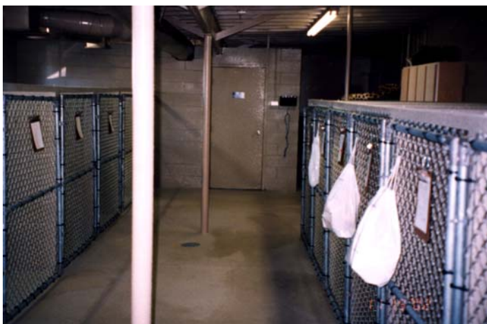
Ranchwood Veterinary Hospital's kennel area after coating application (Courtesy of Sharkskin Industrial Coatings)
