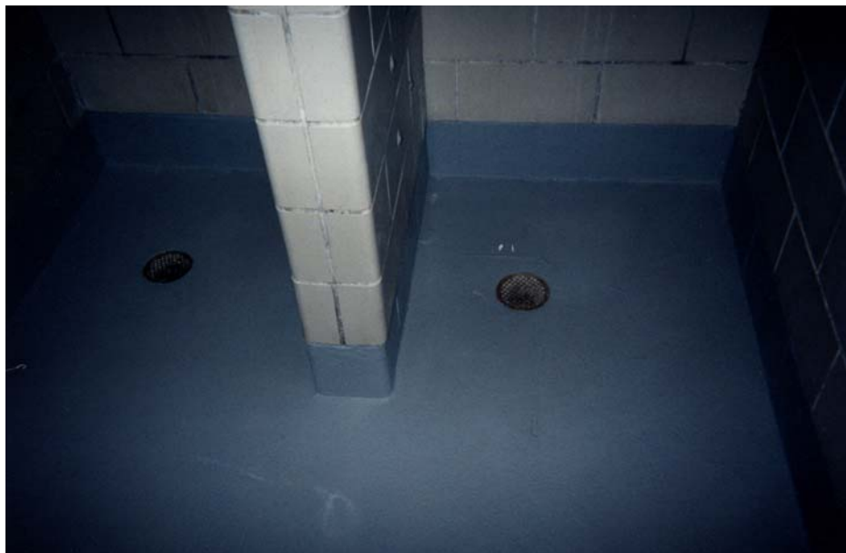
ESI's ElastoGard AL is used as a shower stall coating in a local city park (picture courtesy of Von Castor)
