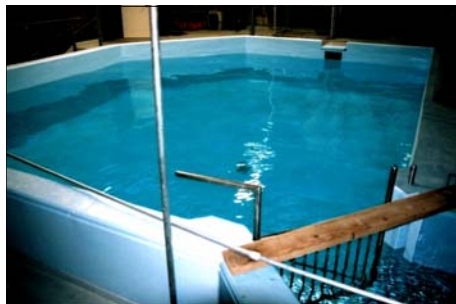
Finished picture of the medicine treatment tank at the OKC Zoo.
